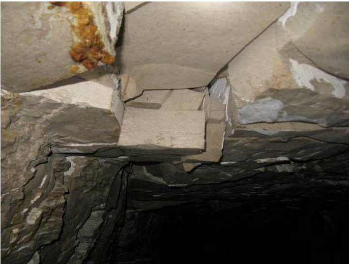
Dangerous rock in the ceiling
